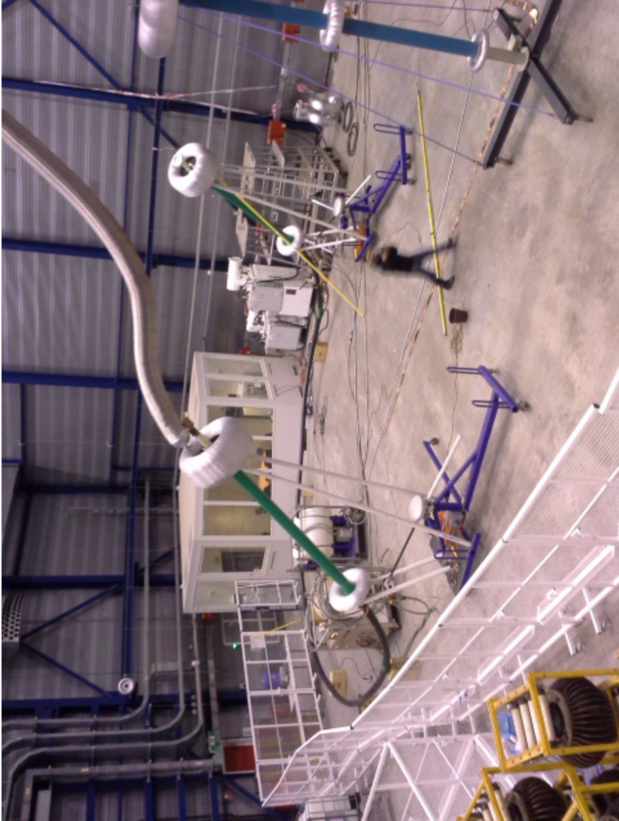
Photograph of the test setup and the cable sample with water terminations installed.
